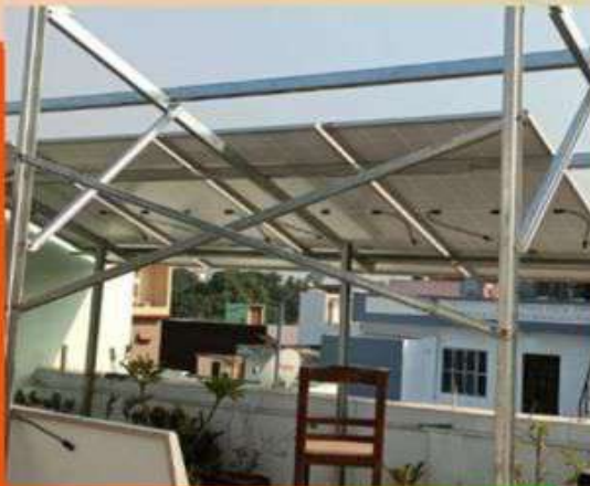
SOLAR POWER PLANT STRUCTURE
